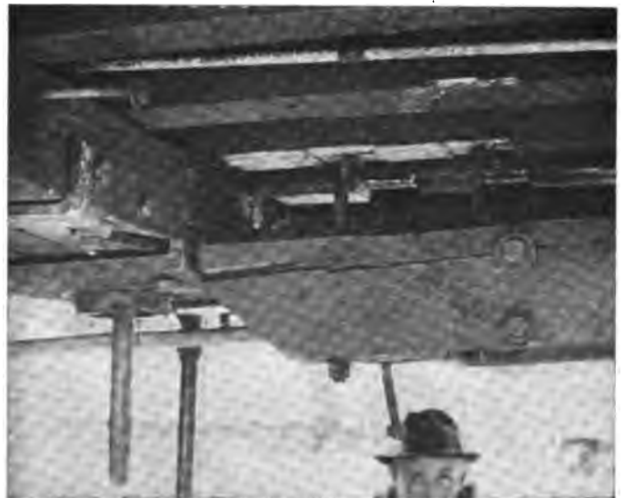
A Common Failure in the Older Freight Equipment.
