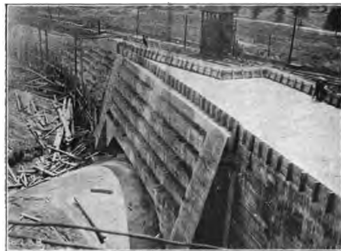
Looking Down on the Wing Wall of the Underjump at Maure Avenue.
