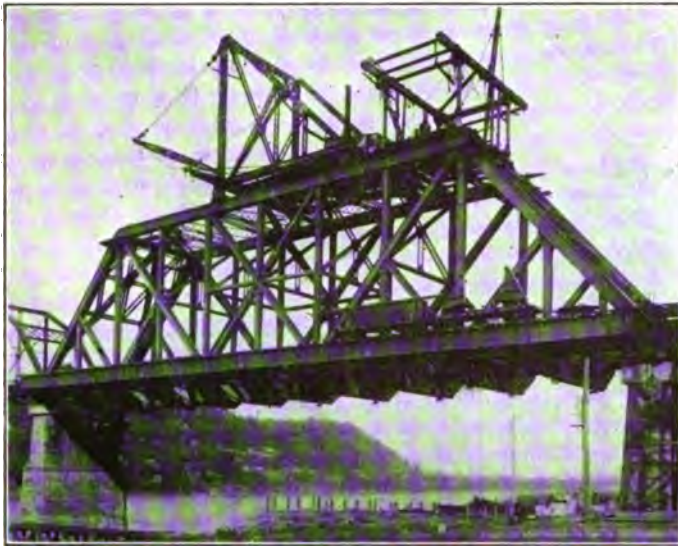
Fig. 8—New Span 1 After Removal of Old Trusses Showing Heavy Traveler Erected for Placing Spans 2 and 3.
