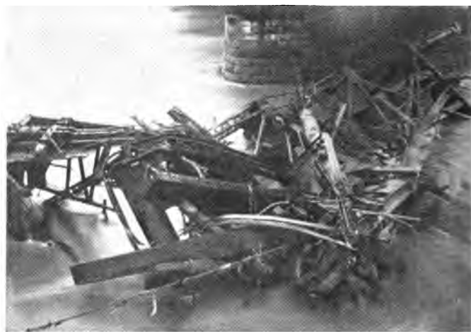
The Wreckage of One of the Spans at Zanesville.
