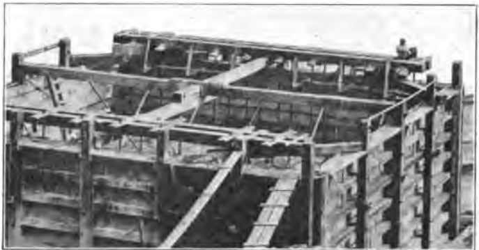
Looking Into One of the Pier Forms, Showing Reinforcement and Form Bracing.
