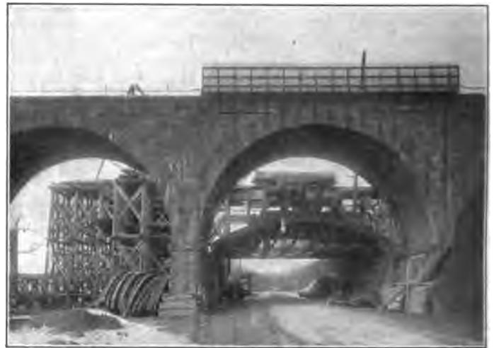
Two of the Old Arches at East End, Showing Material Track and Forms in Place for New Concrete Arches.
