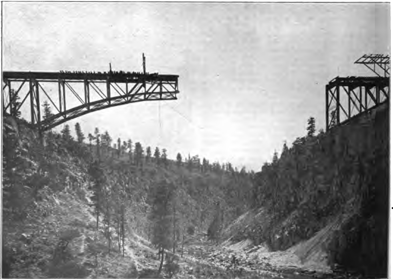
Starting the Erection of the West Half of the Structure. Digitized by Google
