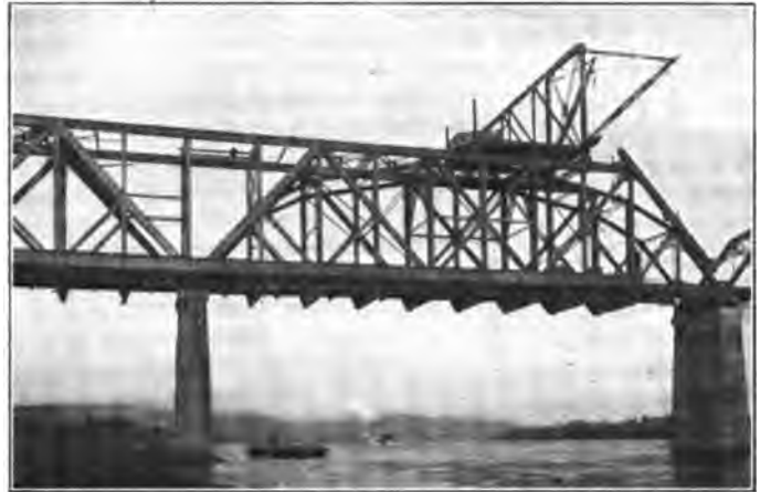
Fig. 11—Placing End Post of Span 2 by Cantilever Method Showing Erection Ties Between Spans 1 and 2.
