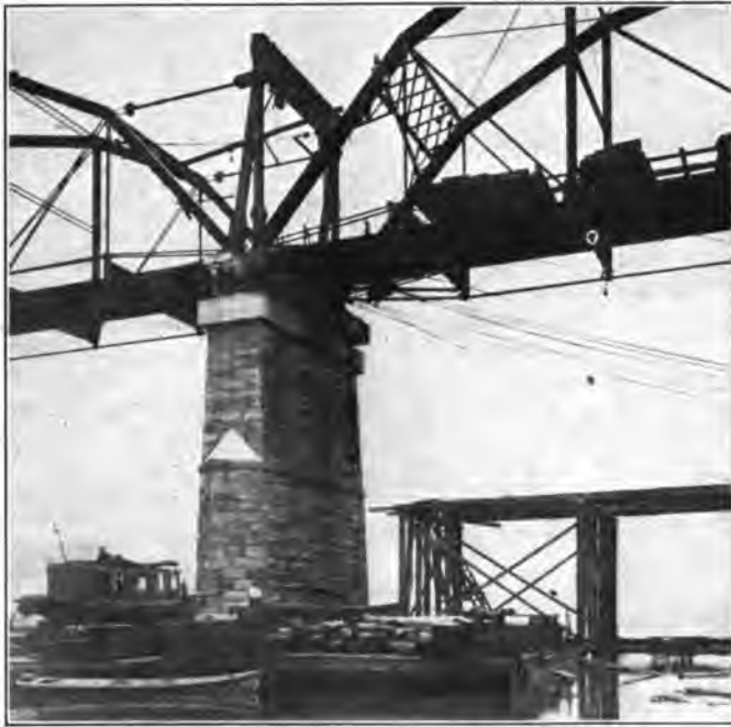
Fig. 3—Placing a Pier Girder Under Old Span after Cutting Away Half of the Top of Old Pier. The Right Hand Span Is Supported Temporarily by the Gallows Frame.
