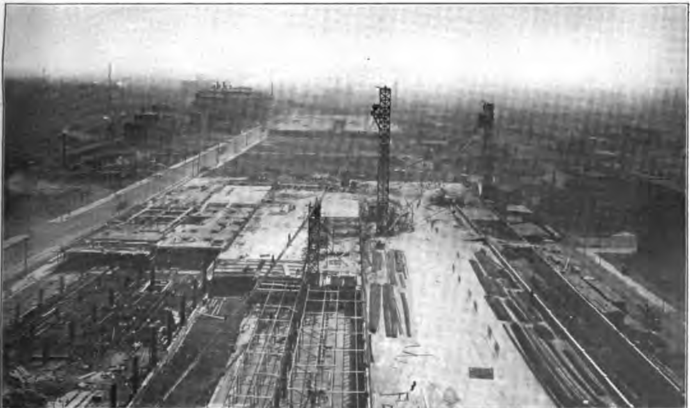
General View of Terminal on July 13. The Three Concrete Plants Are Shown, the One in the Foreground Having One Mixing and Two Distributing Towers.
