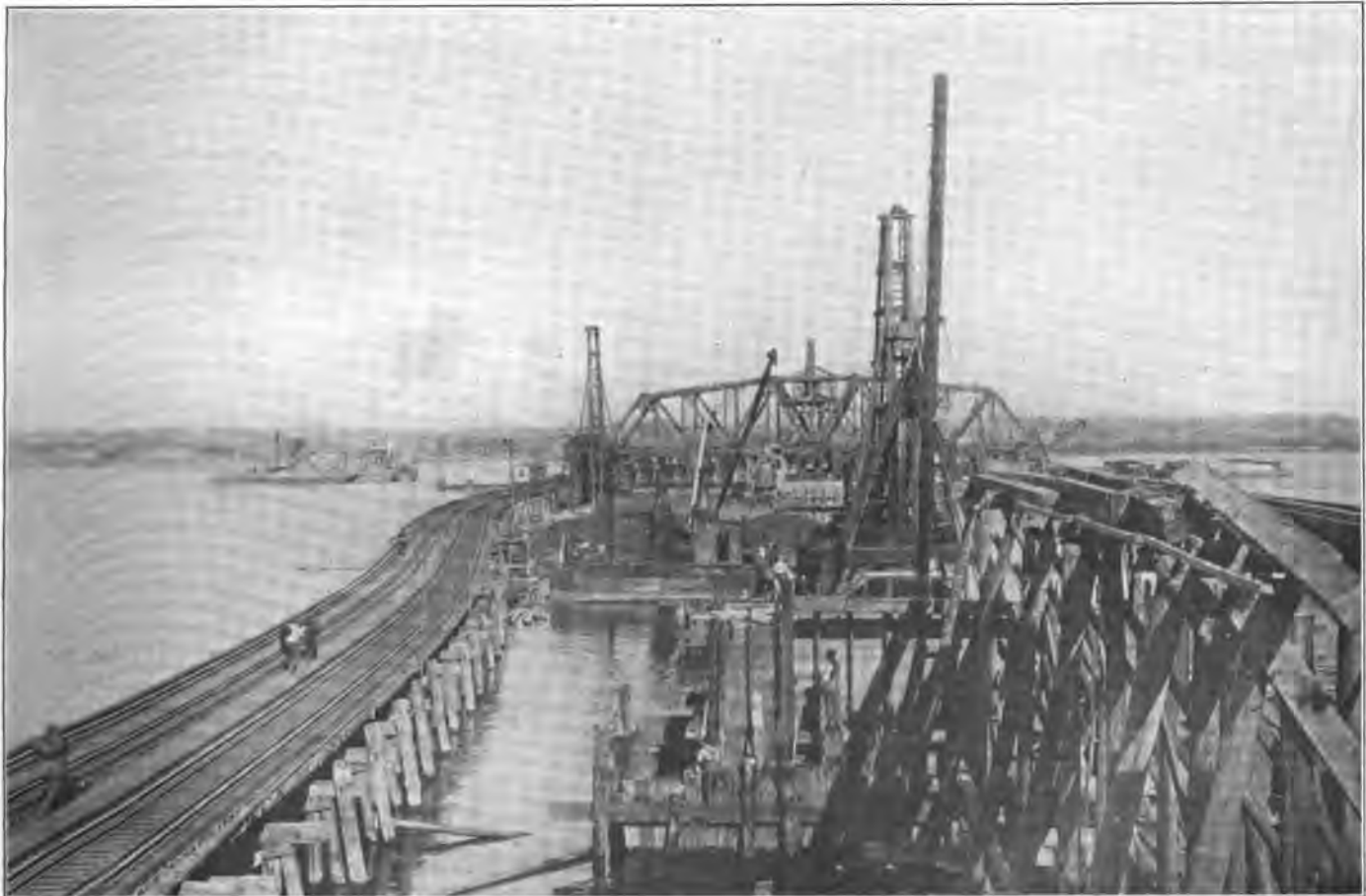
New Hackensack River Bridge Under Construction; Draw Span Erected in Open Position, Piers for West Approach Being Built in Foreground.
