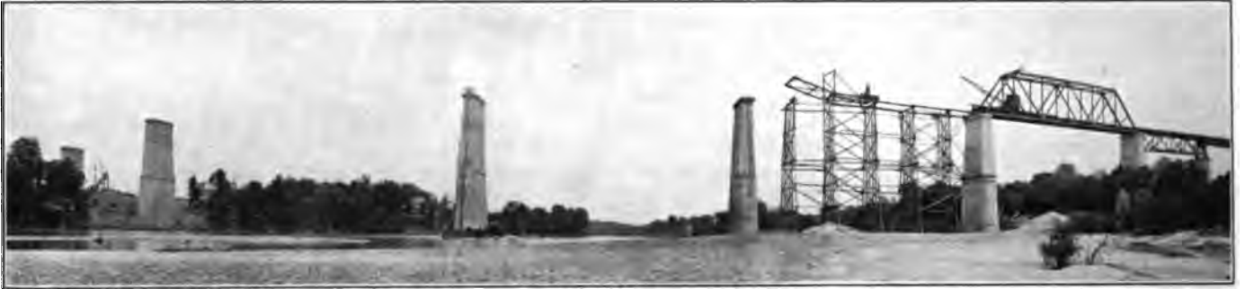
Panorama of Cumberland River Bridge with One Truss Span Erected and False Work Being Placed for the Second.
