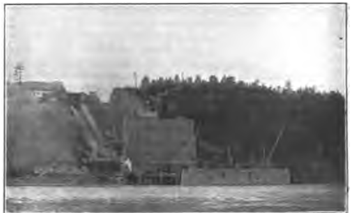
General View of North Side Showing Main and Anchor Piers and Abutment.
