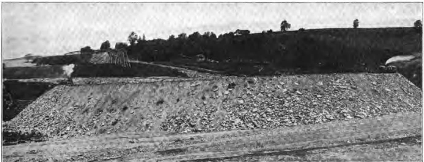
South Branch Fill, Showing Balanced Incline to Lower Lift and Upper Level Trestle.
