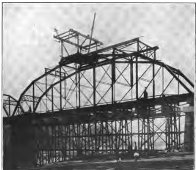
Fig. 7—Old Span 1 Showing False Work Carrying Traffic and Small Traveler Erected on Old Trusses to Place New Span.
