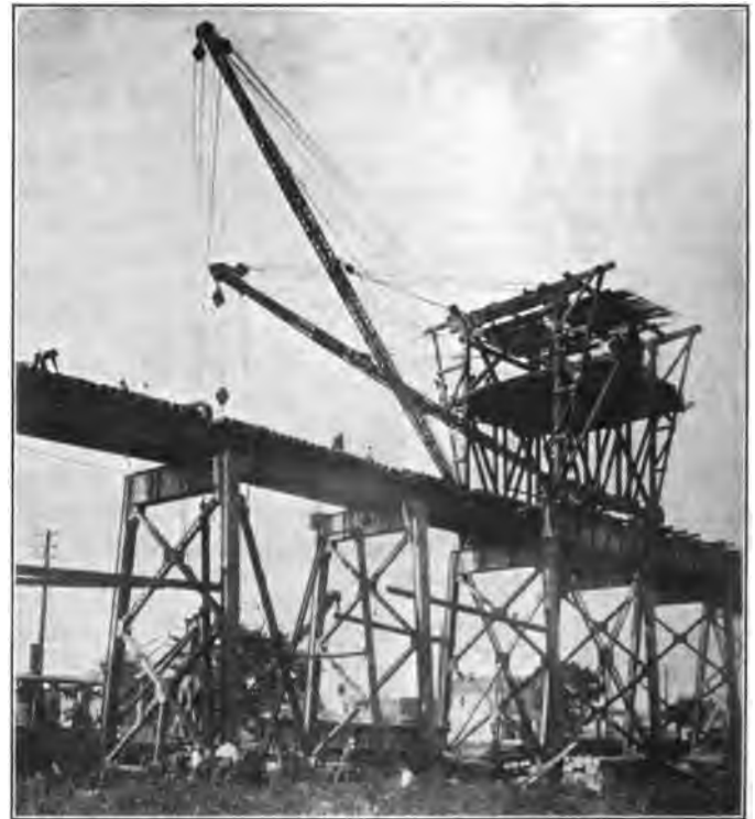
Fig. 14—Erecting New Double Track Viaduct and Removing Old Members Without Interruption to Traffic.
