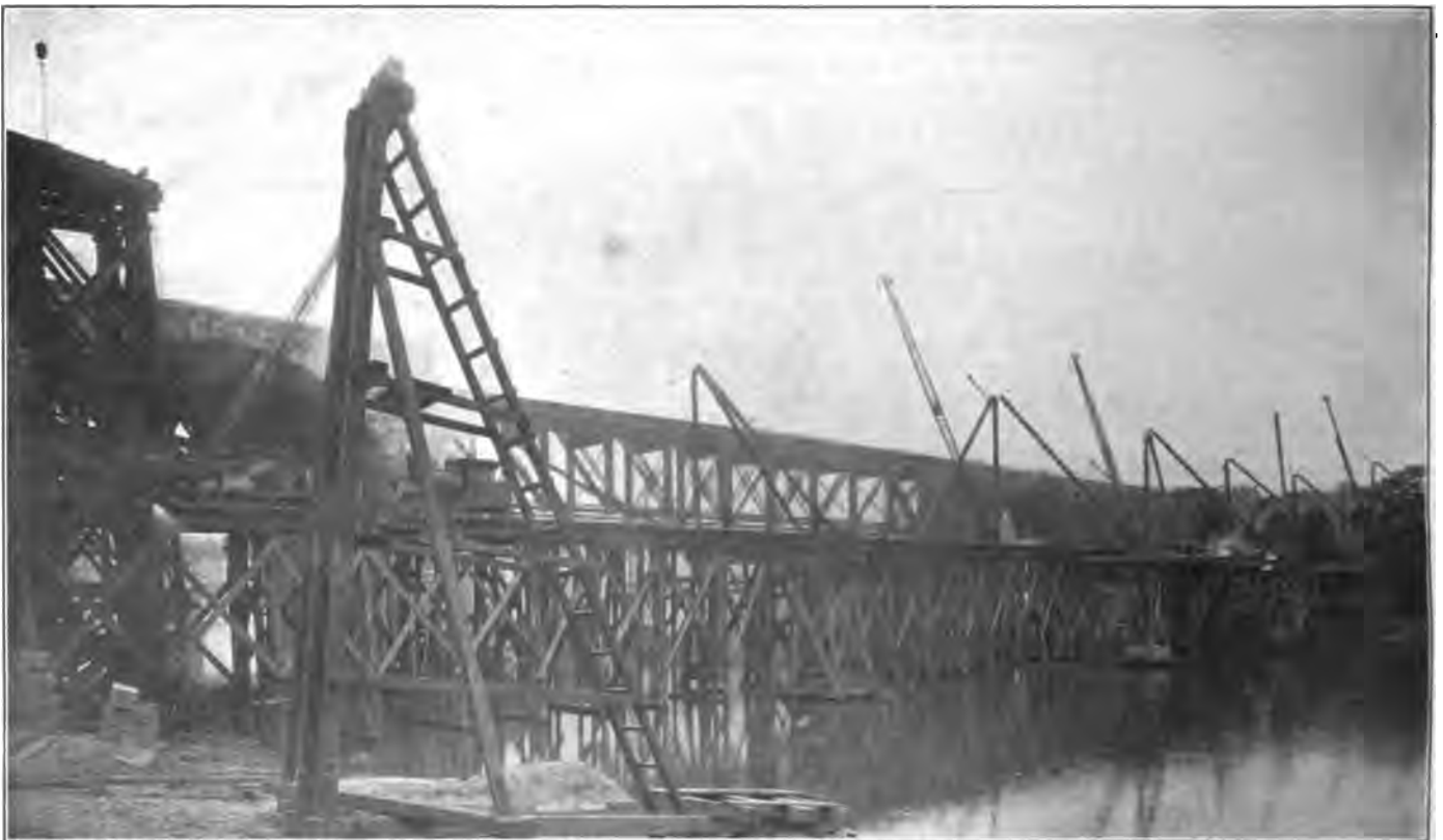
Low Level Trestle Across River from Which Concrete and Stone Were Placed.
