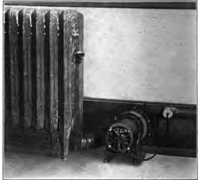
Arrangement of Motor Driven Ventilating Set at a Radiator.
