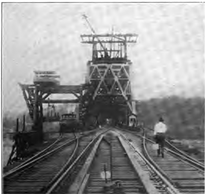
Fig. 6—End View from South Showing Material Tracks and Electric Hoist for Raising Materials to the Bridge from the Ground.
