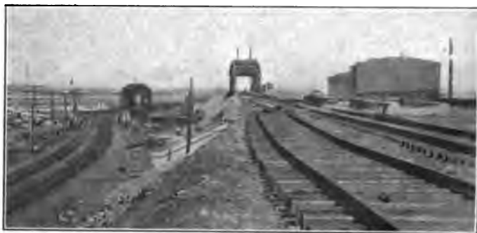
The New Line Across the Passaic River, Showing Temporary Line to Left.
