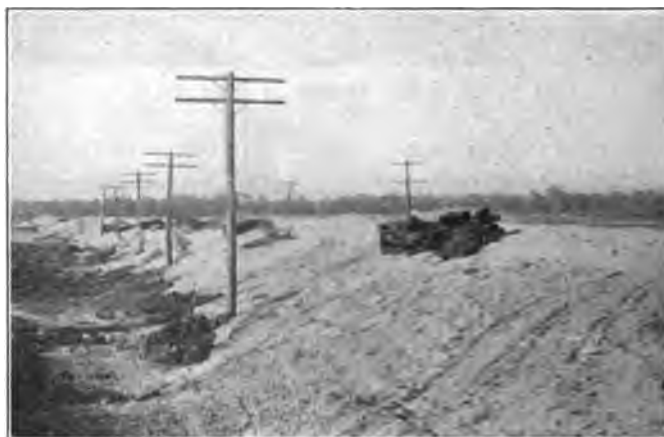
Fig. 4—Embankment Across Wabash River Lowlands Restored to Its Former Elevation. Rails and Ties from the Overturned Track Piled on the Shoulder.
