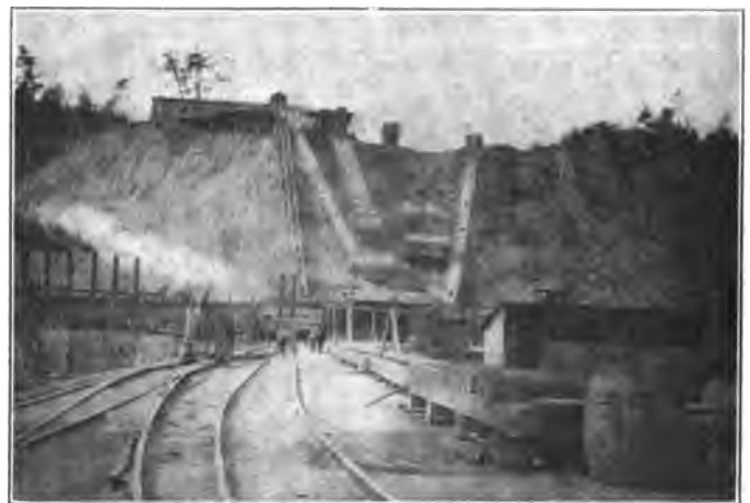
General View of Boiler Compressor, and Mixer Plant on North Side.
