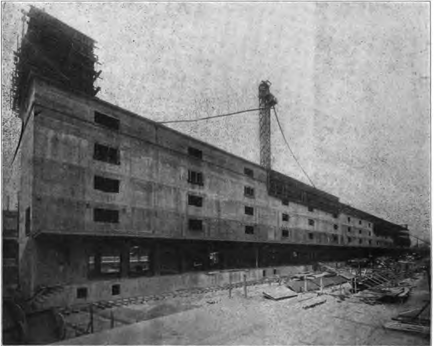
South End of New Freight Station During Construction, Showing Forms and Concrete Distributing Tower.
